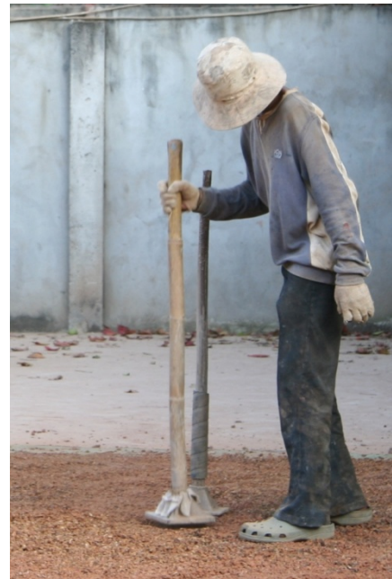
Figure 3.1 Laterite is crushed using Elephant's Foot Tamper and added to RDIC's clay mix
